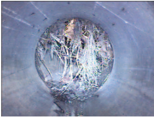
Water pipe with clogged roots
