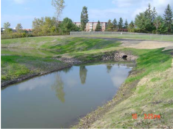
Sediment forebay at Farrell Street Stormwater Detention Pond. To ensure the effectiveness of the pond, sediment collected in the forebay must be removed on a regular basis. Photo taken during construction
