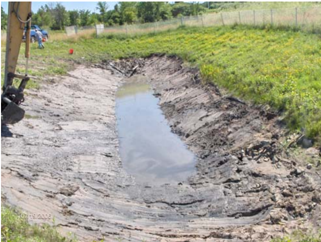
Sediment removal from Bartlett Bay Stormwater Treatment Wetland forebay. Prior to removing the accumulated sediment, the forebay is drained to prevent discharges of sediment laden water to the Stormwater Treatment Wetland.
