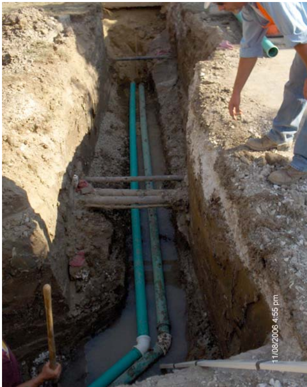
New sanitary pipe was connected to the sewer and existing foundation drain left in place
