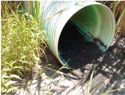
Outfall pipe where sanitary connection was discharging
