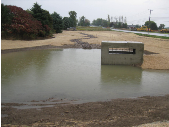
Oak Creek Village extended detention micropool during construction. Permanent pool and outlet structure are visible in the foreground. Stone-lined pilot channel visible in background.
