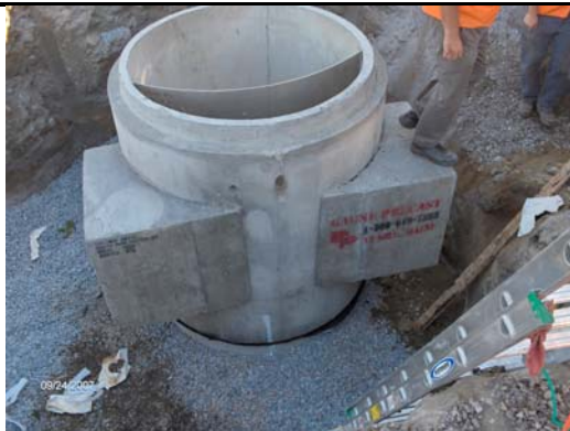
View of swirl separator interior plates.
