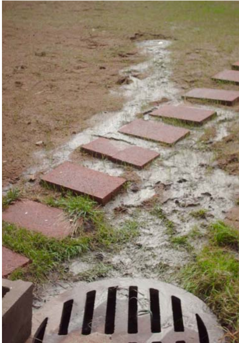
Wastewater bubbling to the surface and flowing into a storm drain
