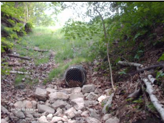
New stormwater outflow
