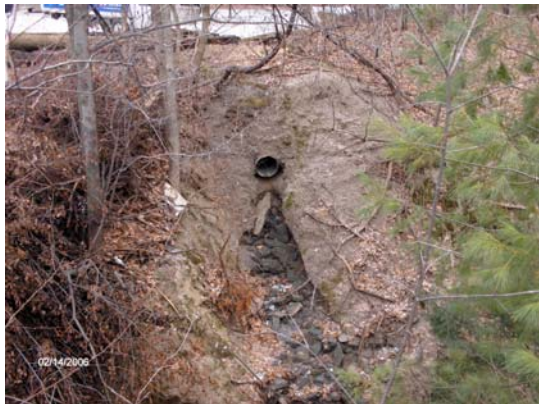
Discharge pipe before the project
