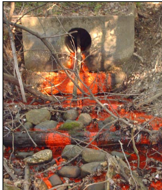
Outfall where dumped field paint discharged to surface waters
